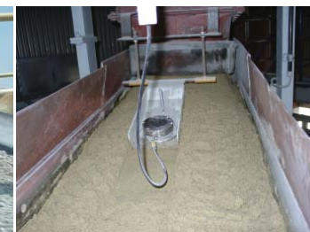
Litronic-FMS II Planar Sensor installed in a sliding shoe for quartz sand.
